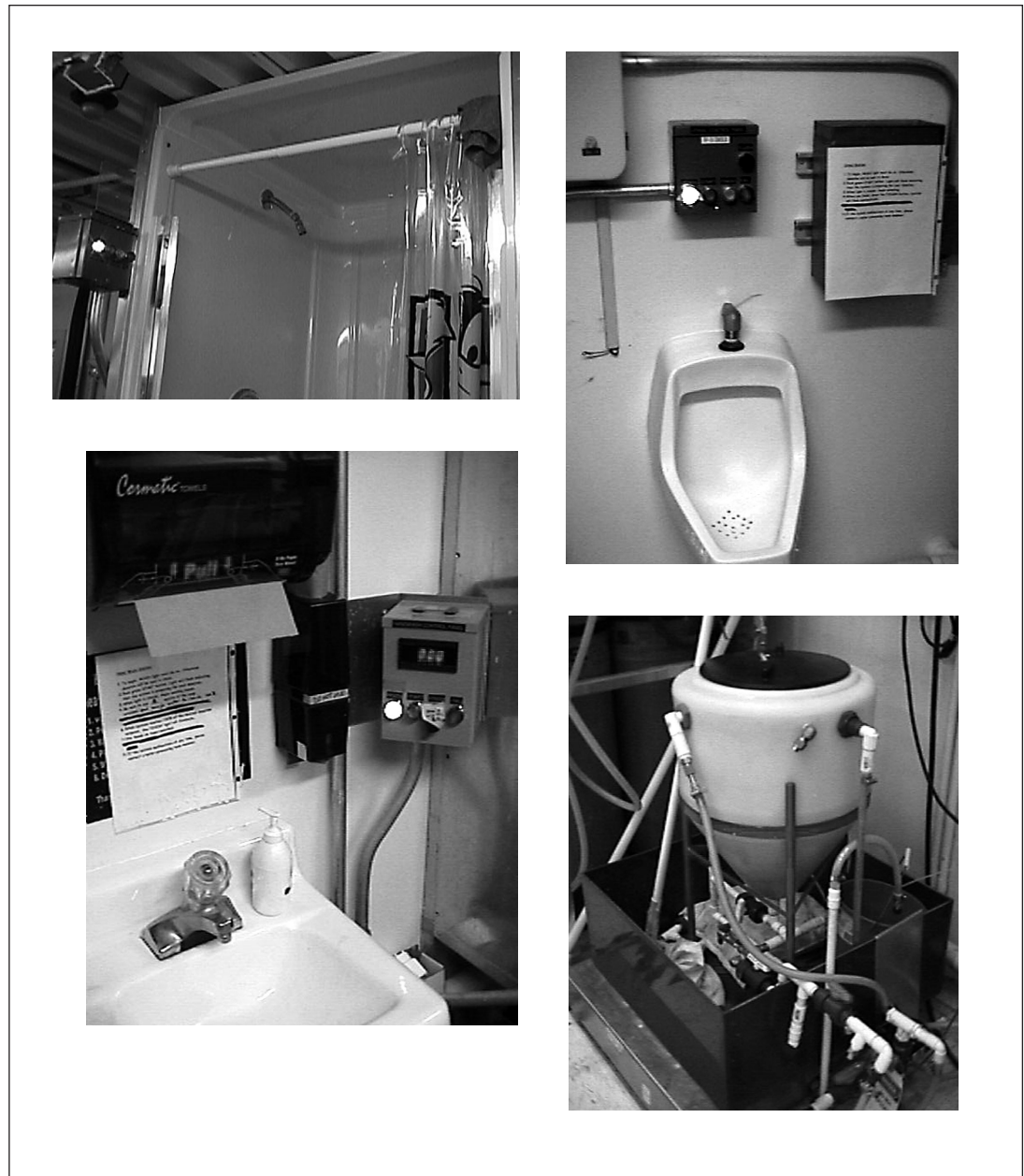
Figure 3. The Integrated Water-Recovery System Waste-Water Collection System.
